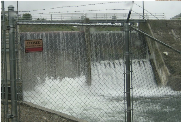
Figure 10. The original dam and powerhouse (B&W) and the rebuilt dam (color, 2002). Low level outlets are indicated and combined operation of the low level outlets and main gate shown.
